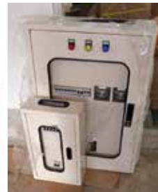
Pump Control Panel
