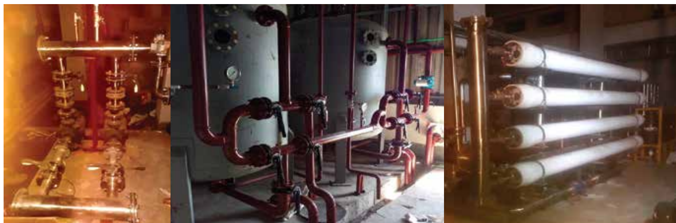
Booster Pumping System
