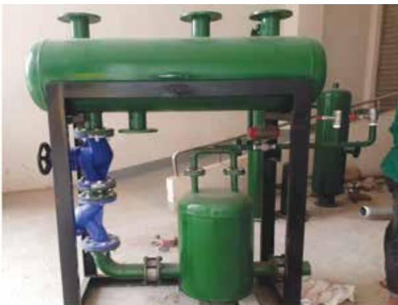
Condensate Recovery Pump
