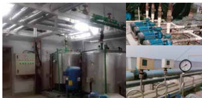
Hot Water System (Geyser System)
