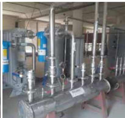
Compressed Air piping
